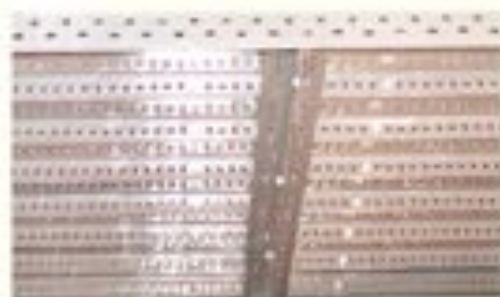
Lower view of floor grating
